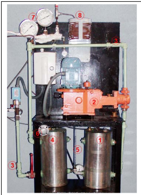
Figure 6 - Water supply system with water feed pump, pressure vessel and Steam condenser.
