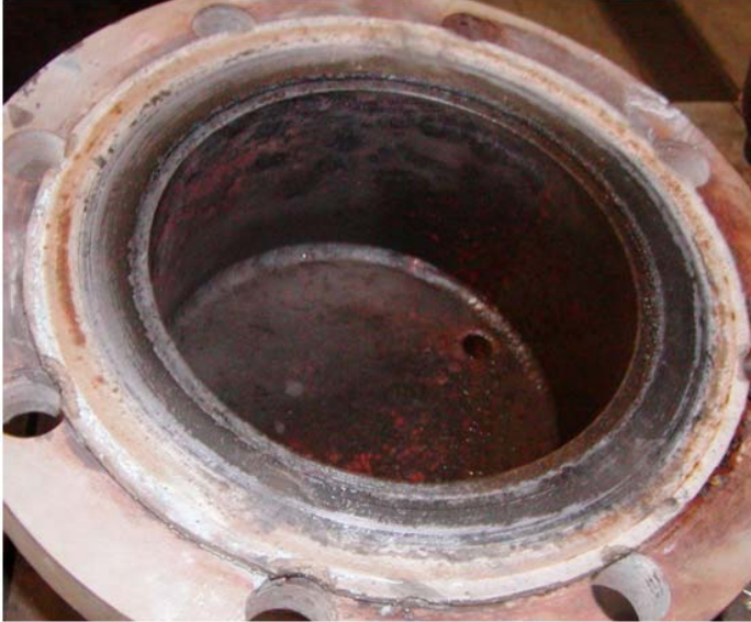
Figure 4: Teadit NA1122 after test.
