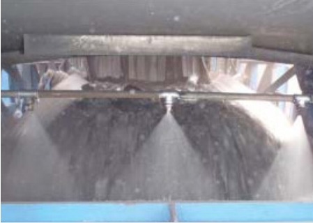
Conveyor Head Box Sprays
