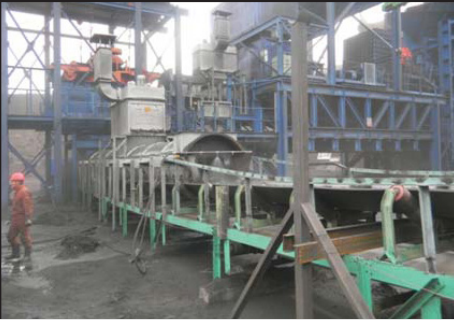
Conveyor Transfer Point
