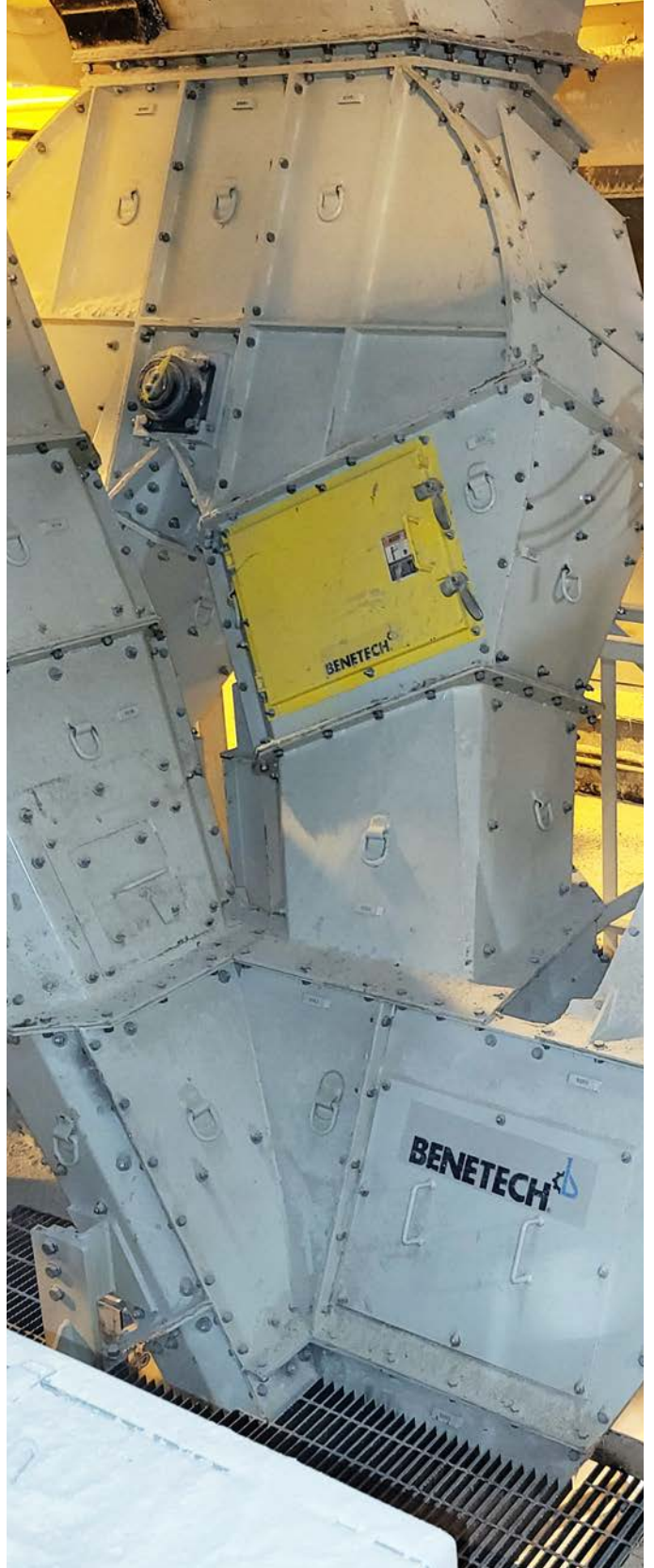
Transfer Chutes After
